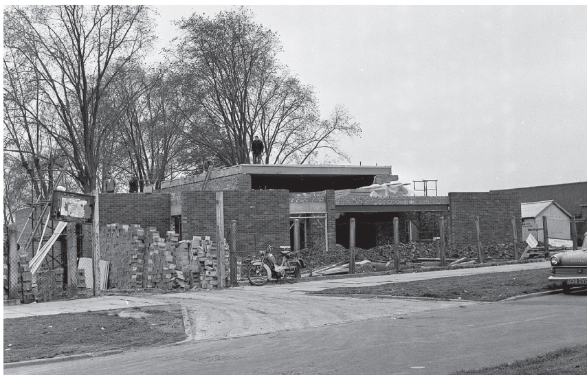
(ABOVE) Stocking Farm Youth Club under construction (1968) in the soon to be Community Shop.
